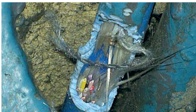
Nagerschaden an Kabel / Rodent damage to a cable
